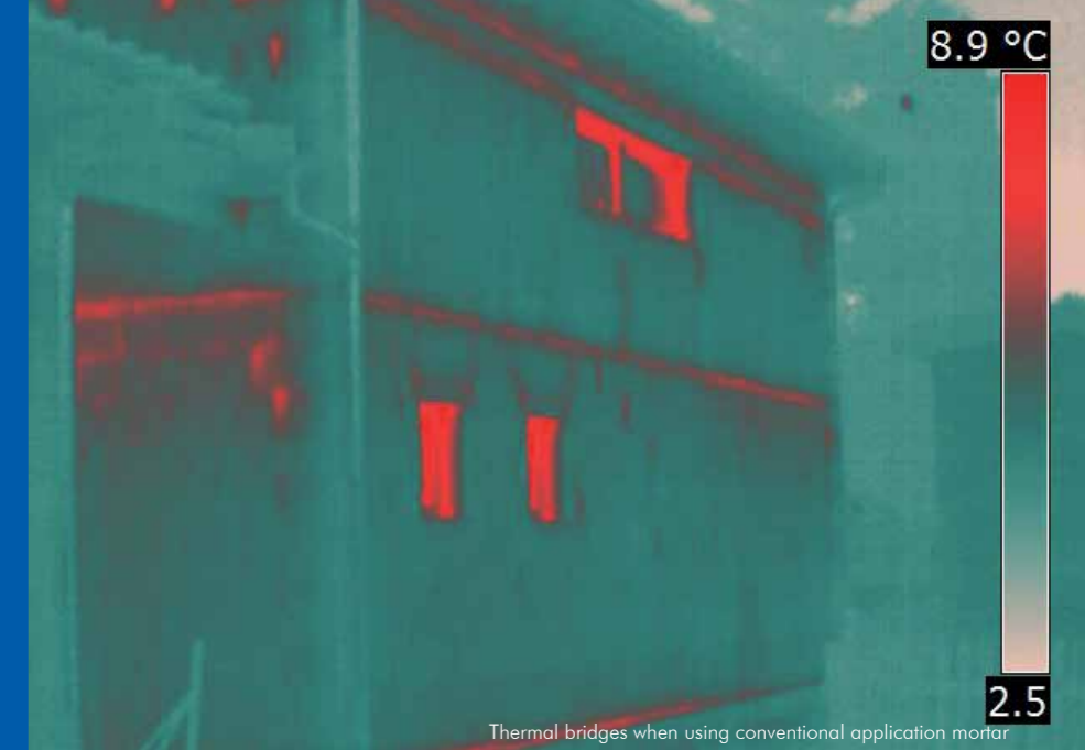
Thermal bridges when using conventional application mortar
