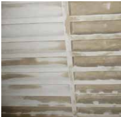
Reprofiled ribbed ceiling
