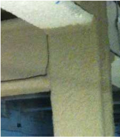
Sprayed structural steel section left unfinished
