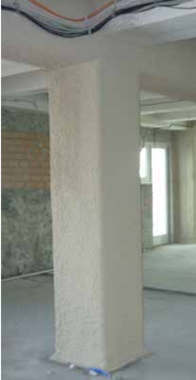
Sprayed concrete column left unfinished
